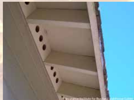
Open-eaves and eave-vents are particularly vulnerable to flames and embers.
