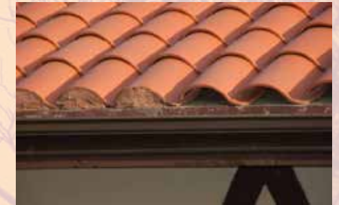
Only 1/2 of the tiles shown in this image have bird-stops installed. Embers may ignite debris beneath the exposed tiles.
